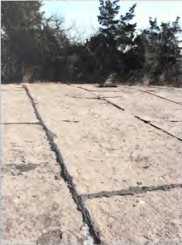
Figure 3.35. Close-up view of concrete terreplein, Battery Granger. The concrete terreplein shows evidence of an asphalt-based product either used to fill joints or remaining in the joints after use as part of a larger concrete surface treatment (Olmsted Center, January 2009).
